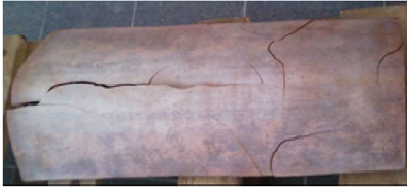
Fig. 12 Different and very deep clefts and cracks lesions within the tile.
